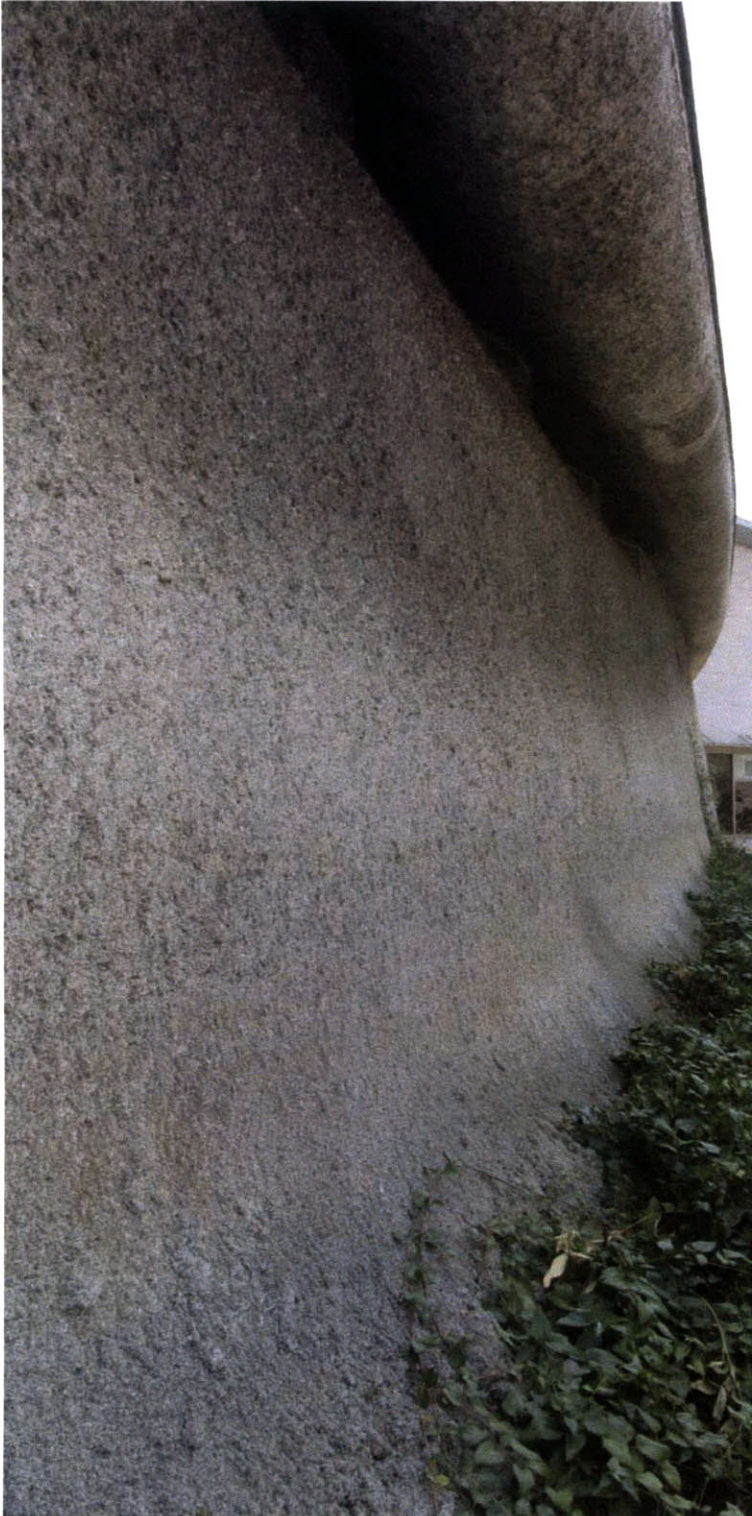
Figure 5.15 Wall details of Takarazuka Catholic Church (1966) showing sprayed mortar surface. Hyogo, Japan Architect: Murano Togo Photograph taken by author.
